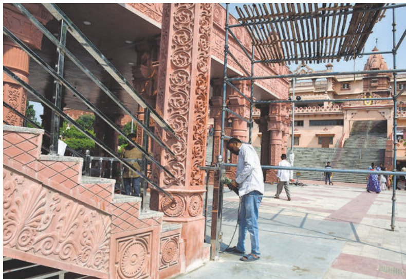
Green plans: Work under way at a visitors' shelter near the Krishna Janmabhoomi Temple at Mathura in Uttar Pradesh. R. V. MOORTHY
